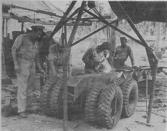
Outside of the tires, not one bit of new materials went into "Lowboy's" construction. Chief Machinist's Mate A. Vincent Spencer, extreme left, supervised the job.
